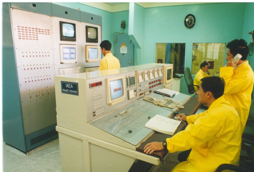
The control room of the DNRR
