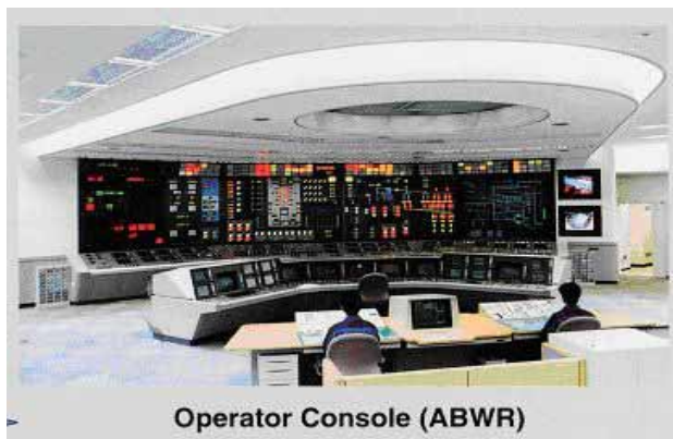
Fig. 12-1 Main Control Panel of ABWR
