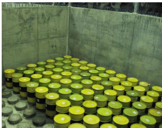
The Combined Storage and Repository for Low and Medium Level Radioactive Waste in Himdalen (Photo: NRPA)
